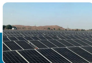
Solar Ground Mount
