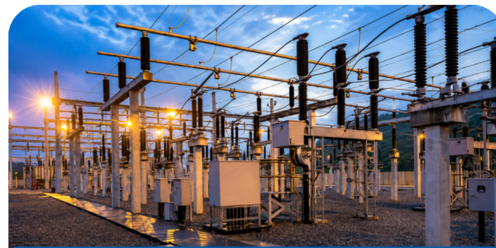
Upto 400KV/60+ Substation
