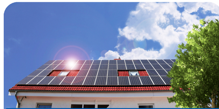
120+ MW Residential Solar Rooftop
